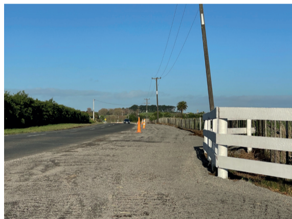
Good progress is being made on the Normanby-Hāwera pathway. The pathway, which is part of the Council's pathway programme, will run along Katermarae Road and connect with the Glover Road pathway.
